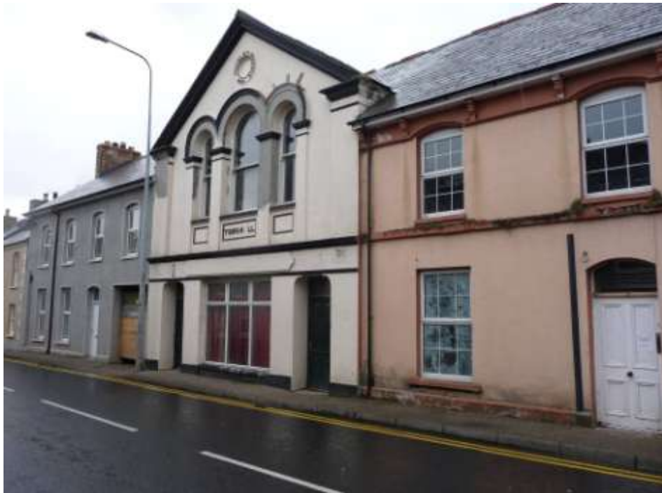
Figure 227 – replacement of timber windows to Town Hall with plastic and cement render repairs, Newtown Stewart
