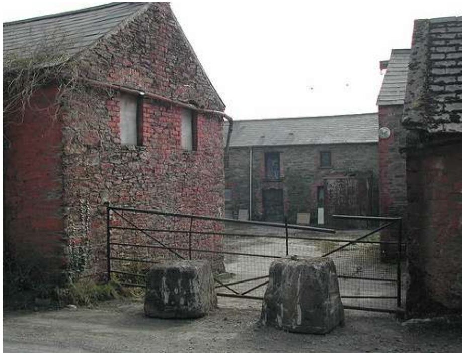
Figure 308– Dairy and outbuildings HB01/27/018 Ballyarnett; important example of vernacular farm buildings falling into disuse (c) UAHS
